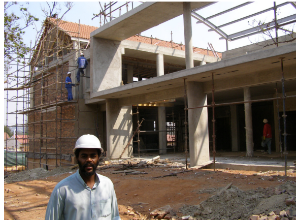
Barrow Construction's Mike Makhudu pictured at the entrance to the new St Mary's Waverley Performing Arts centre
